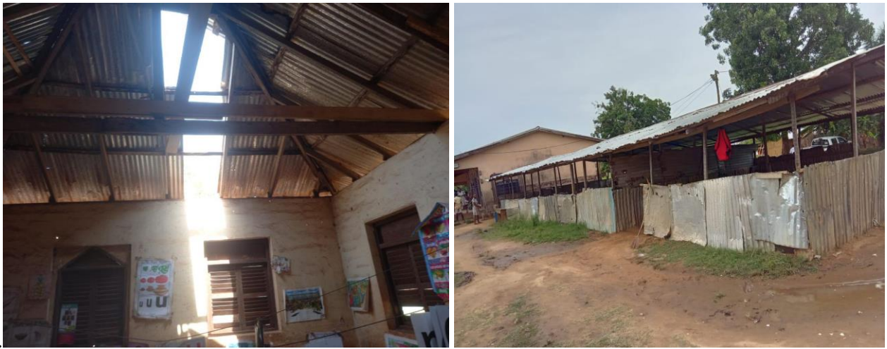
Figure 1: Classrooms in deplorable state. Findings shown in Figure 2 revealed that besides the school building being in a poor and deteriorating state, several classrooms were faced the problem of insufficient furniture. This resulted in the children using bench-like furniture as makeshift tables and chairs, while others resorted to using dual desks.
